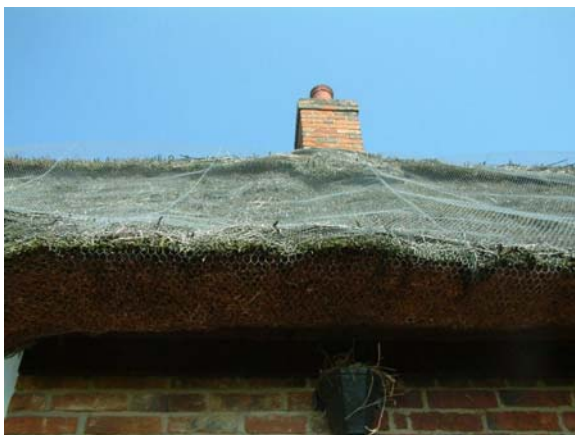
Dips in the thatch, visible spars and loose netting are all signs that a roof requires attention
